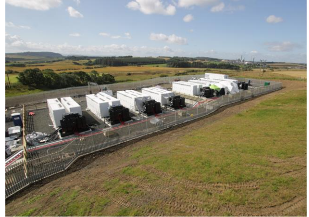
The Company's Little Raith project (49.5 MW / 99 MWh) in Fife, Scotland, which is nearing energisation
