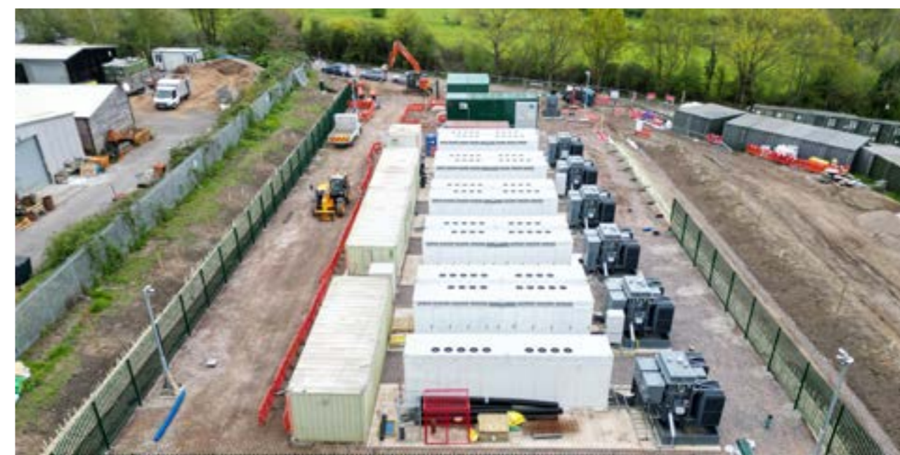
Energised in May 2023, the 20 MW / 40 MWh Farnham Project is the third to be energised in the Company's portfolio.
