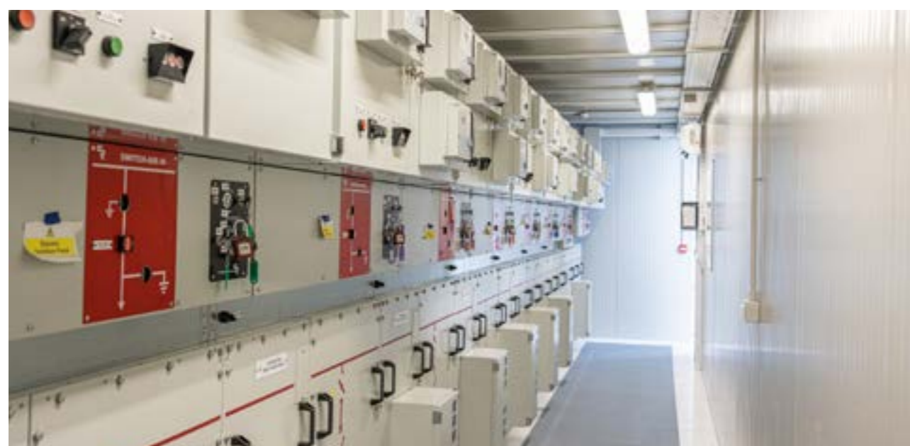
A shot of the control room of the Pillswood project, tracking one of GB's best performing BESS of 2023.
