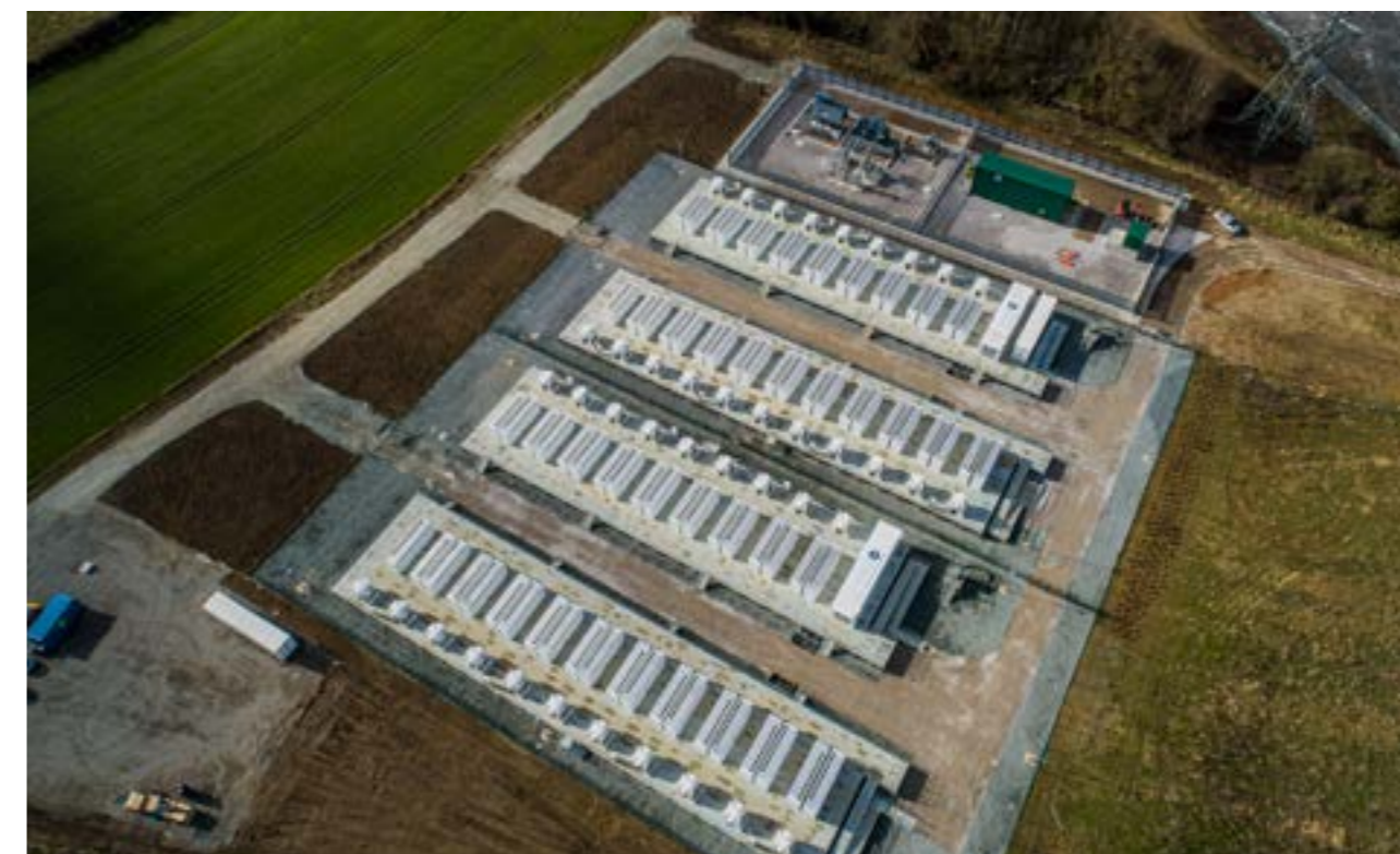
Aerial view of the Company's Pillswood site, Europe's largest BESS by energy capacity (98 MW / 196 MWh).
