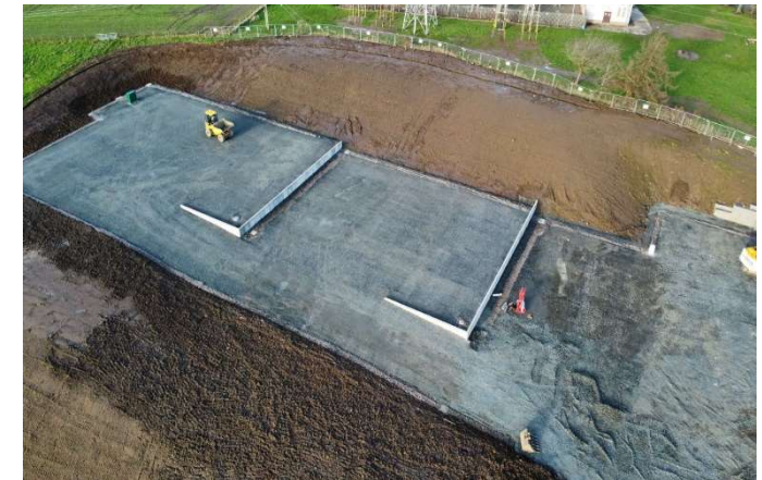
LITTLE RAITH 49.5MW / 99MWh TARGET COD: Q4 2023
