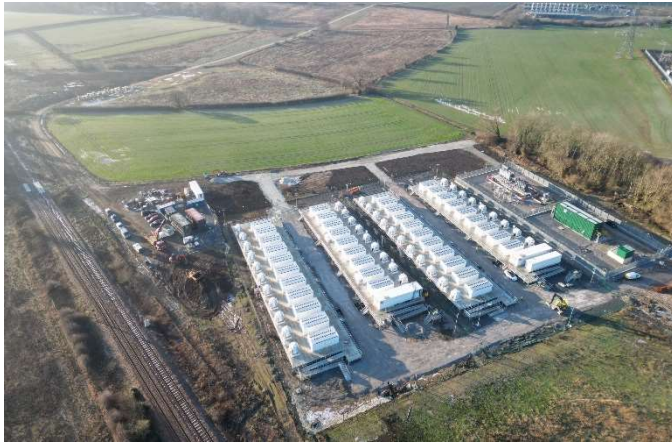
PILLSWOOD 98MW / 196MWh OPERATIONAL
