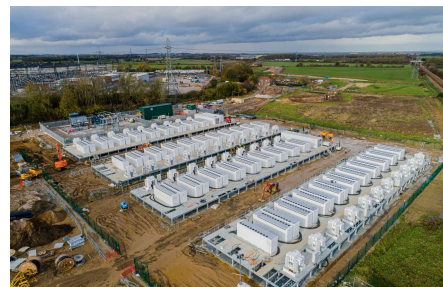
The Company's Pillswood project (98MW/196 MWh), in final preparation for energisation (9 Nov 2022)
