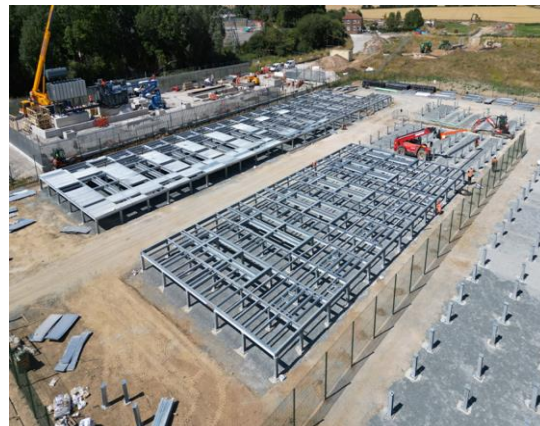
The Company's Pillswood Project (98 MW / 196 MWh). Steel platforms being prepared to receive delivery of the Tesla Megapacks, the first batch of which are expected on site before end August 2022
